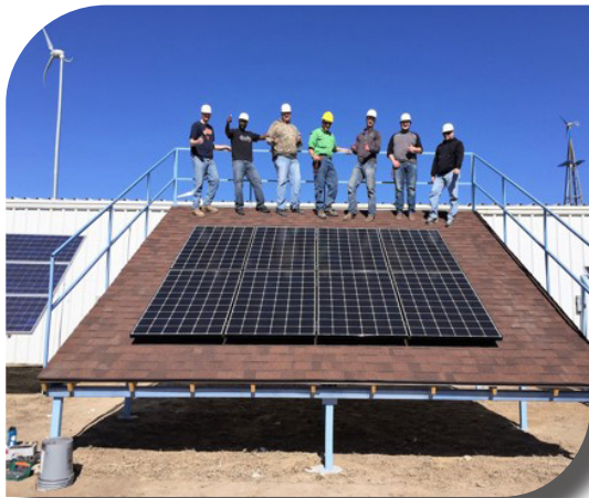
Students installing solar panels on a mock rooftop during a Saturday boot camp.
