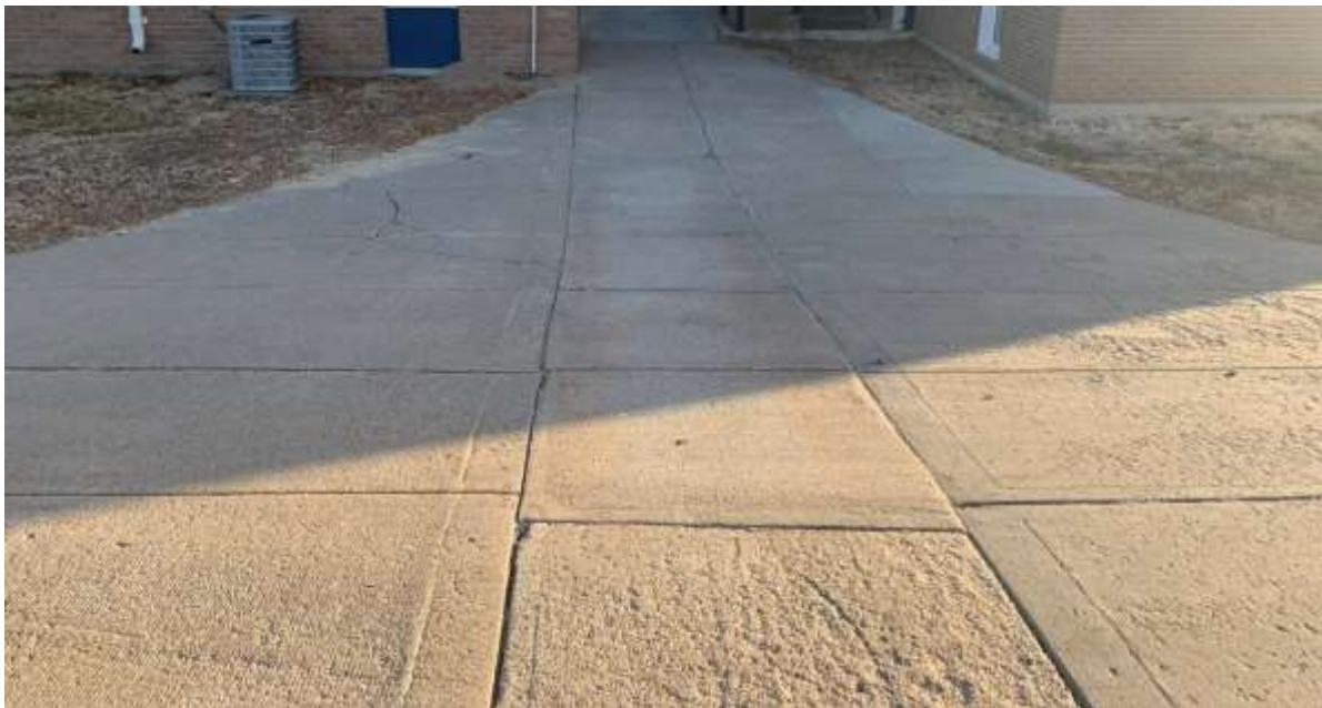
South Hines Hall Entrances Sidewalk, approximately 700 sq. ft.
